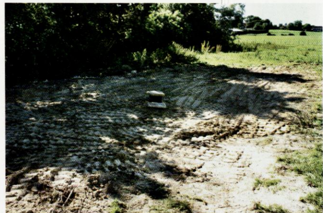
October 2010 – Rob, me, Jon Barker, Nick Pedley and an inquisitive chicken examine the problem with the air intake shaft (which is the second biggest leak). The demolition crew only vaguely lined up the capping slab with the shaft when they broke out the supporting
